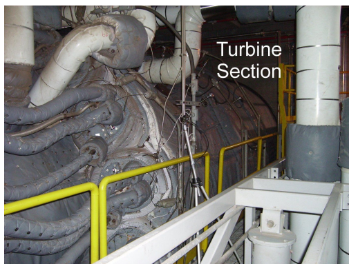
Figure 8: View of the turbine section of the gas turbine
